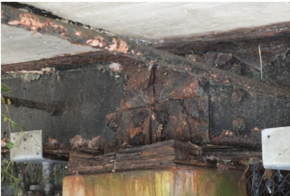
Typical corrosion at support locations.
