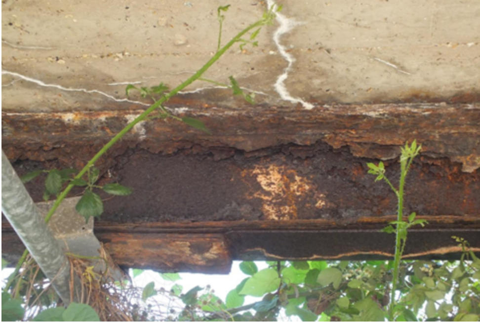
Typical corrosion underneath the ramps.
